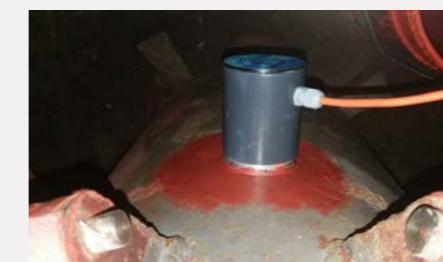
Transducer installed on side of strainer
